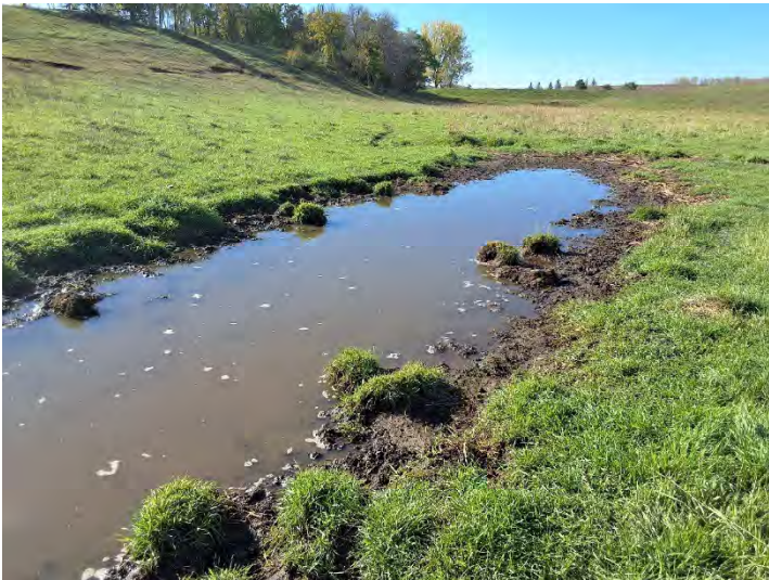
Pooled water observed in the ephemeral channel/swale drainage system.
